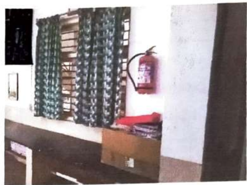
Figure 18 - Placement of Fire extinguisher.
